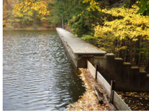
Upper Mine Hill Reservoir Dam - Concrete Deterioration on the Upper Portion of Upstream Face of Dam
