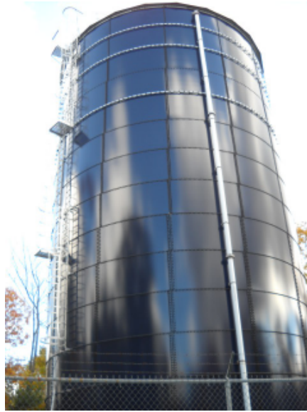
Independence Township Water Storage Tank
